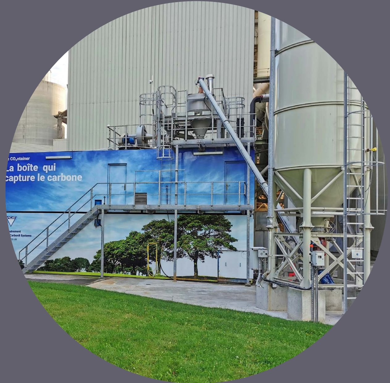
Photo: The CO 2 ntainer at Vicat Group's cement plant in Montalieu, France. In 2020, Carbon8 deployed its Plug 'n Play solution to the cement plant as the first commercial deployment of the containerised system.
